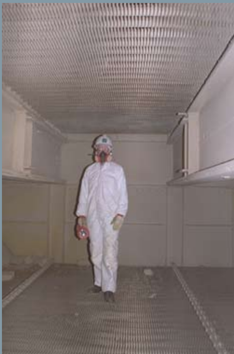
Economiser after firing on coal (water washed)
